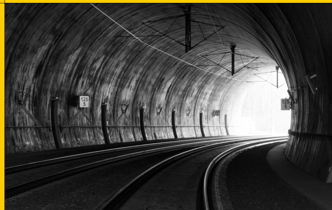
ŽELEZNIČNÍ TUNEL TOMICE II NA TRATI VOTICE-BENEŠOV TOMICE II RAILWAY TUNNEL ON THE VOTICE-BENEŠOV LINE
